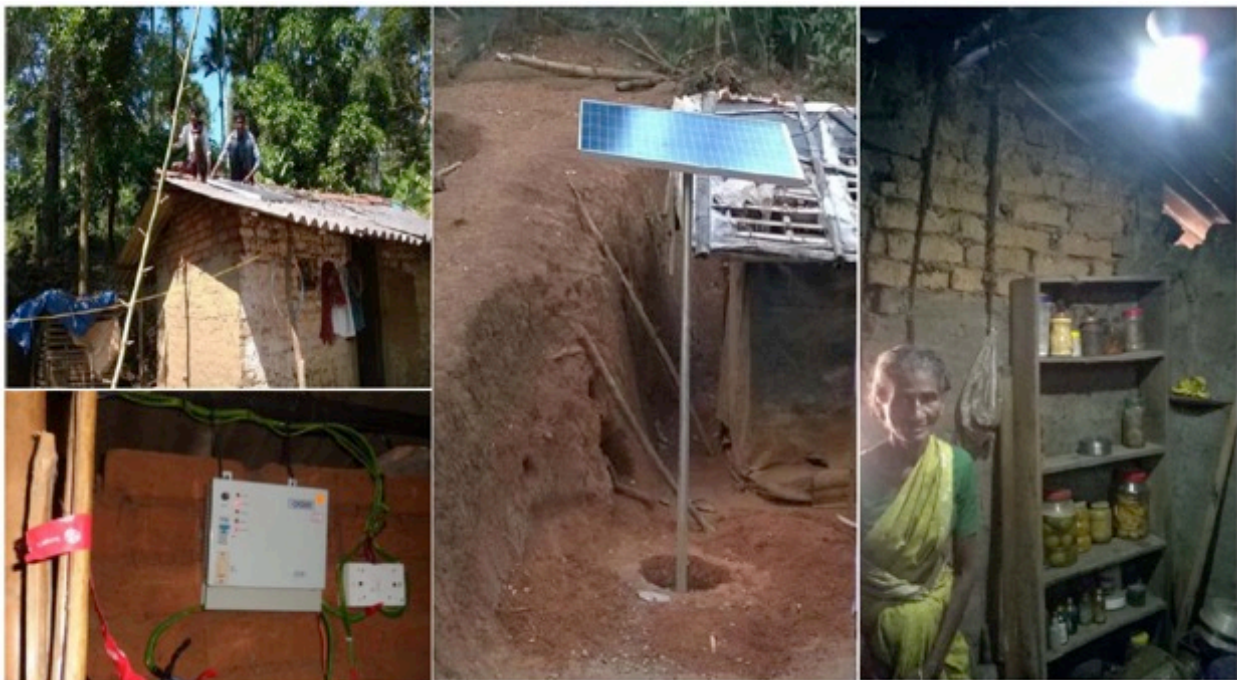
Figure 3: Solar panel installations (top left and middle) and direct current appliances supported through Verizon and Sasken corporations as part of their CSR obligations.
